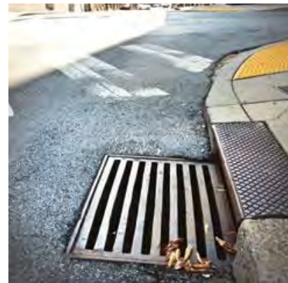
A bicycle-unfriendly sewer grate design in Nashville, TN. These should be avoided at all costs.;
